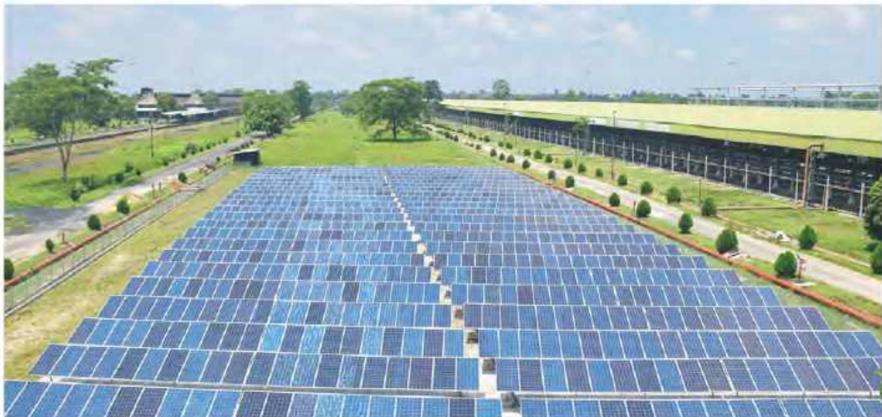
1MWP solar power panels spread inside Numaligarh Refinery is a move towards renewable energy usage
