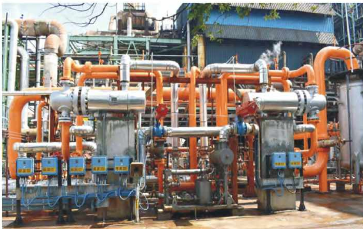
RLNG – Pressure Reducing Station at CPCL, Manali Refinery
